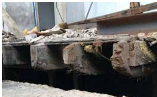
Wood Damaged by termites and rot
