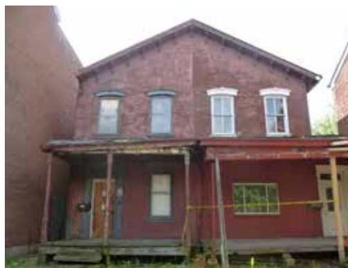
Leaning Beam caused by unstable or undersized posts
