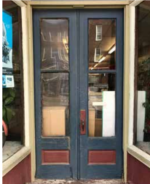
Historic Double Doors constructed with wood and with large panes of glass
