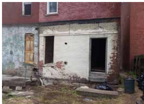
Decaying Mortar Joints create structural instability
