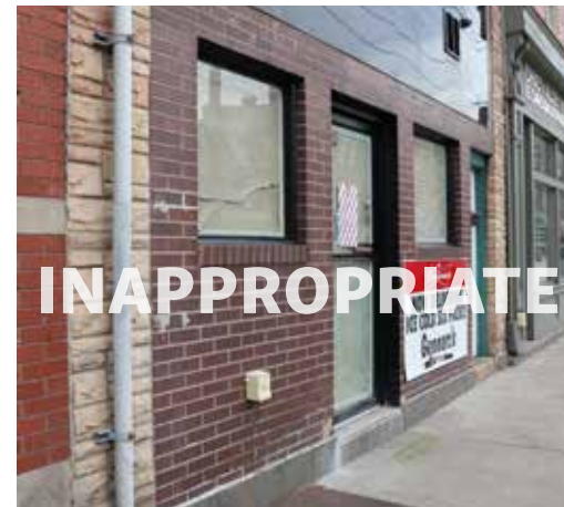
Modern Storefront has inappropriate windows and storefront openings for historic districts
