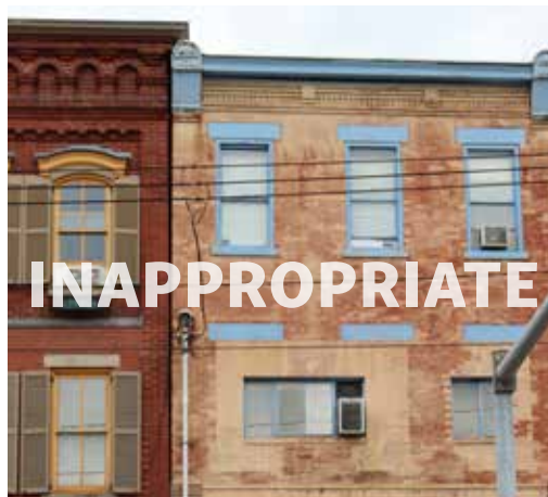
Inappropriate New Windows closed historic openings and have the incorrect size, style, and placement
